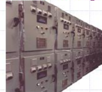
T/R Cabinets, T/R Sets, Diode Stacks, Voltage Dividers and Bushings
